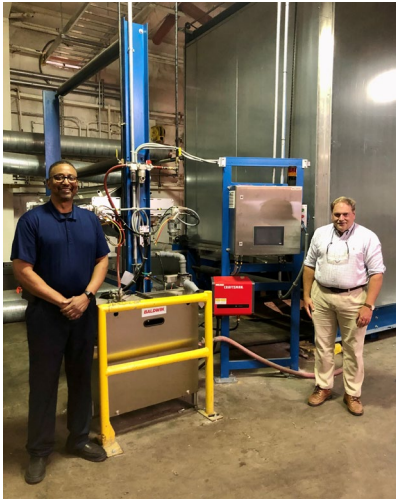
Graniteville Specialty Fabrics team members Bennie Mathis, Plant Superintendent (left), and Doug Johnson, Executive Vice President of Development and Technical Services (right), stand with the newly installed TexCoat G4 from Baldwin.
